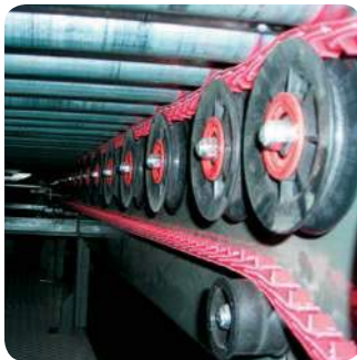
PowerMax V-Belt Idlers used with PowerTwist Roller Drive on a Live Roller Conveyor.
